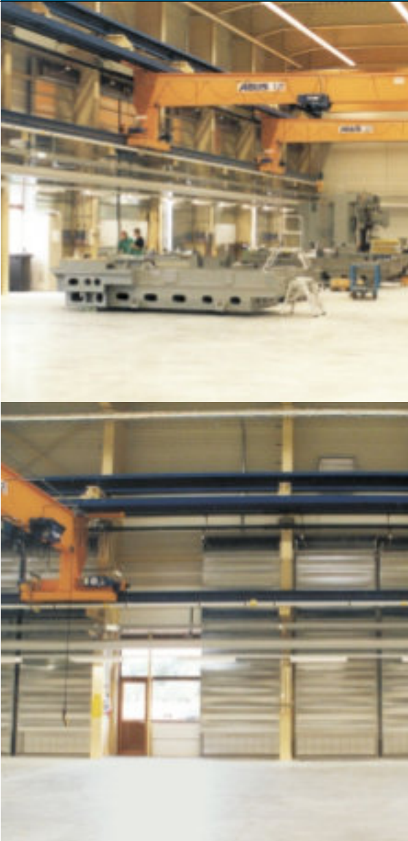
Arrangement of the ADO gTHERM system at the hall's walls provide a flexible utilisation of the hall area
